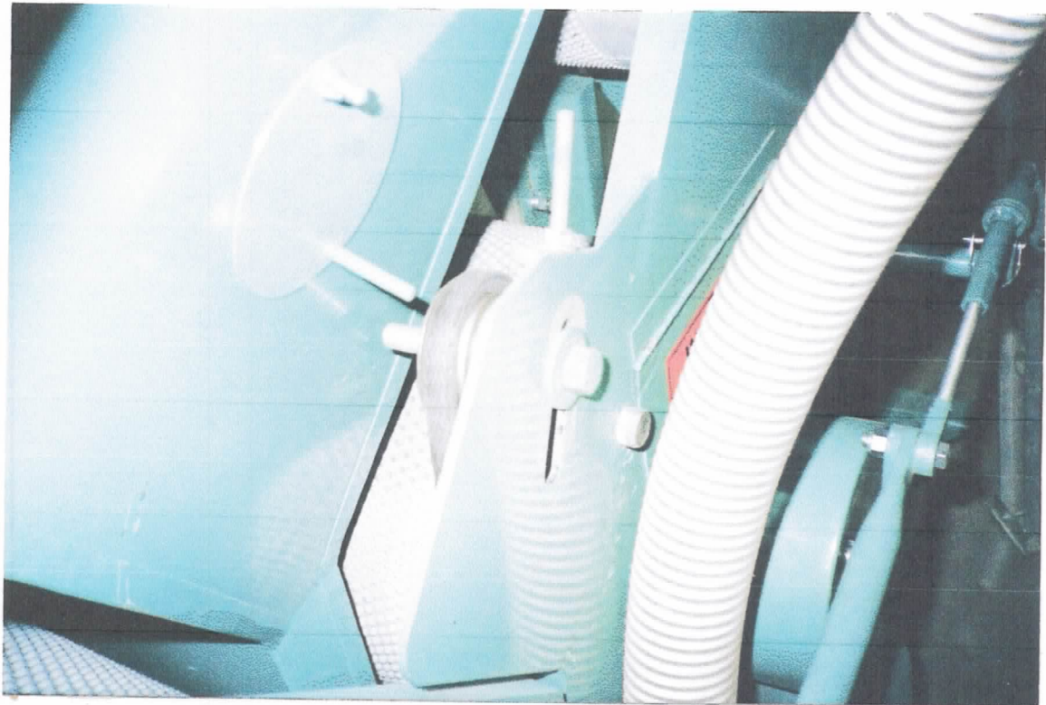
Screenings auger, belt tightener and hopper inspection door.
